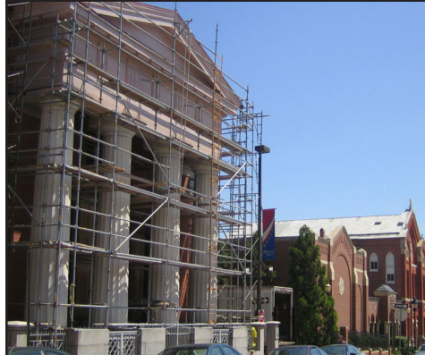
The historic Lloyd Street Synagogue is under renovation. Members will attend the exhibit on the neighborhood's past at the Jewish Museum, to the right, at the corner of Lombard Street.
